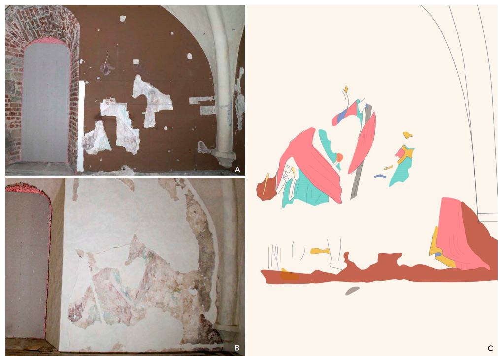
Figure 14. Chapel's fresco on the upper part of the wall. (A) Before restoration (photo: L. Irbeniece, 2020); (B) after conservation. Damaged plaster is conserved and fixed, and the lost areas are filled with lime plaster. On the fresco's surface, there is a historic white haze, still hiding the true colours of the painting (photo: M. Rasiņa, 2021); (C) A sketch of the chapel's fresco showing fragments of the medieval figurative painting (drawing: M. Rasiņa, I. Vanadzīņa, 2021).
