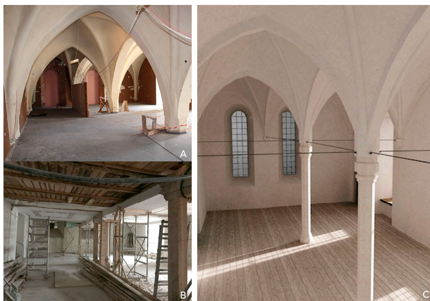
Figure 3. Chapel in Riga Castle. (A) Chapel, upper floor level, before restoration (photo: M. Rasiņa, 2018); (B) chapel, ground floor level, before restoration (photo: M. Rasiņa, 2020); (C) 3D visualization (by architect Reinis Liepiņš, 2015 [1]) of how the chapel will likely look after restoration.
